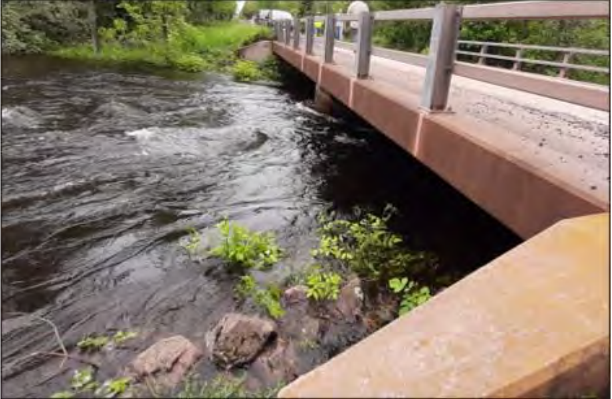
End of Reach 1 – Upstream of South Drive bridge at 1,200 cfs, clearance roughly 3 feet
