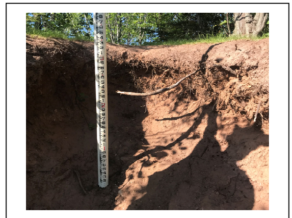
154. Island #35 – Bank erosion
