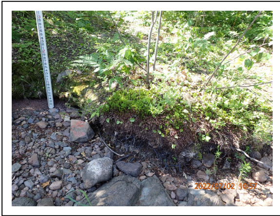
61. Island #13 – Bank erosion
