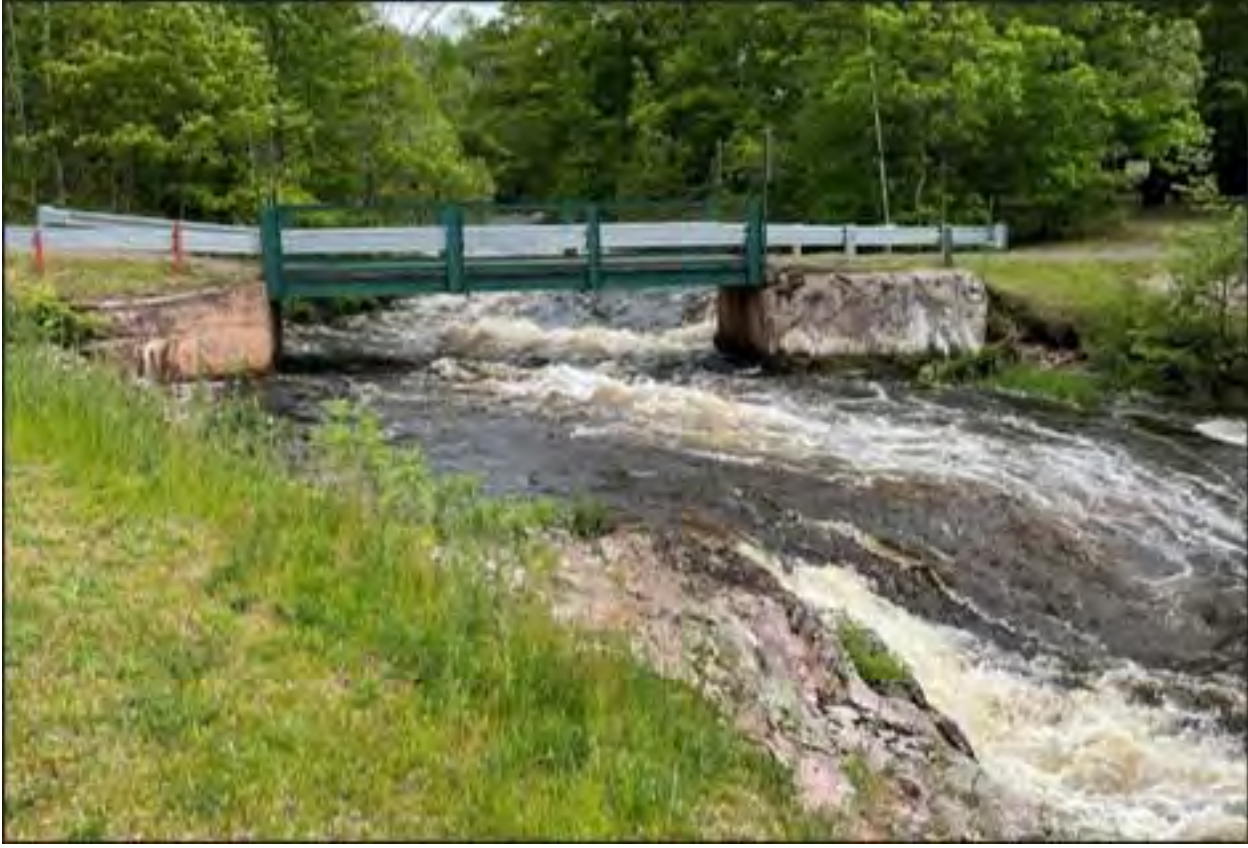
End of Reach 3 – Kimball Town Park bridge downstream of Kimball Falls at 1,200 cfs
