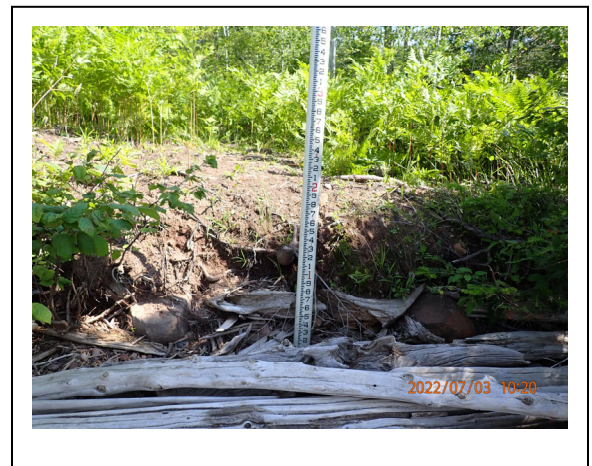
96. Island #20 – Bank erosion
